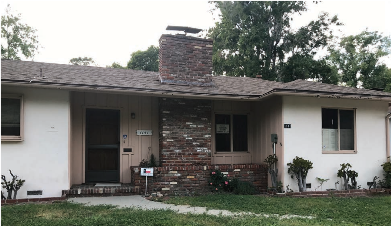
What looks like to be feces smeared on the walls.
