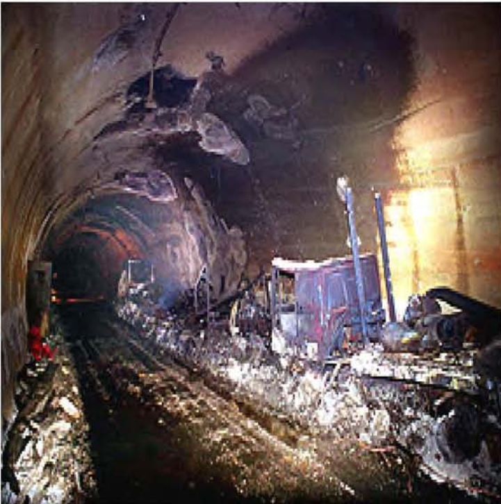
Mont Blanc Tunnel Fire, France/Italy 1999 39 Dead
