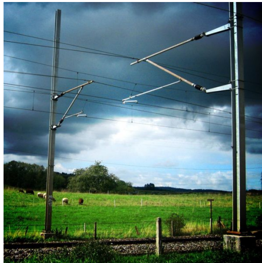
Figure 4 Swiss Federal Railways overhead lines
