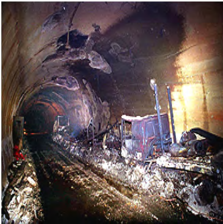
Mont Blanc Tunnel Fire, France/Italy 1999 39 Dead
